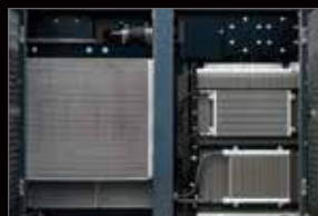
Cooling System Components
